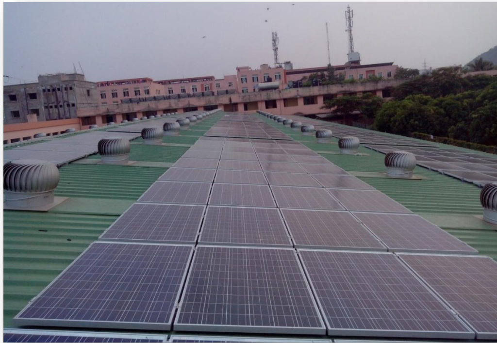
KALINGA INSTITUTE OF SOCIAL SCIENCES 500 KW SOLAR ROOFTOP INSTALLATION
