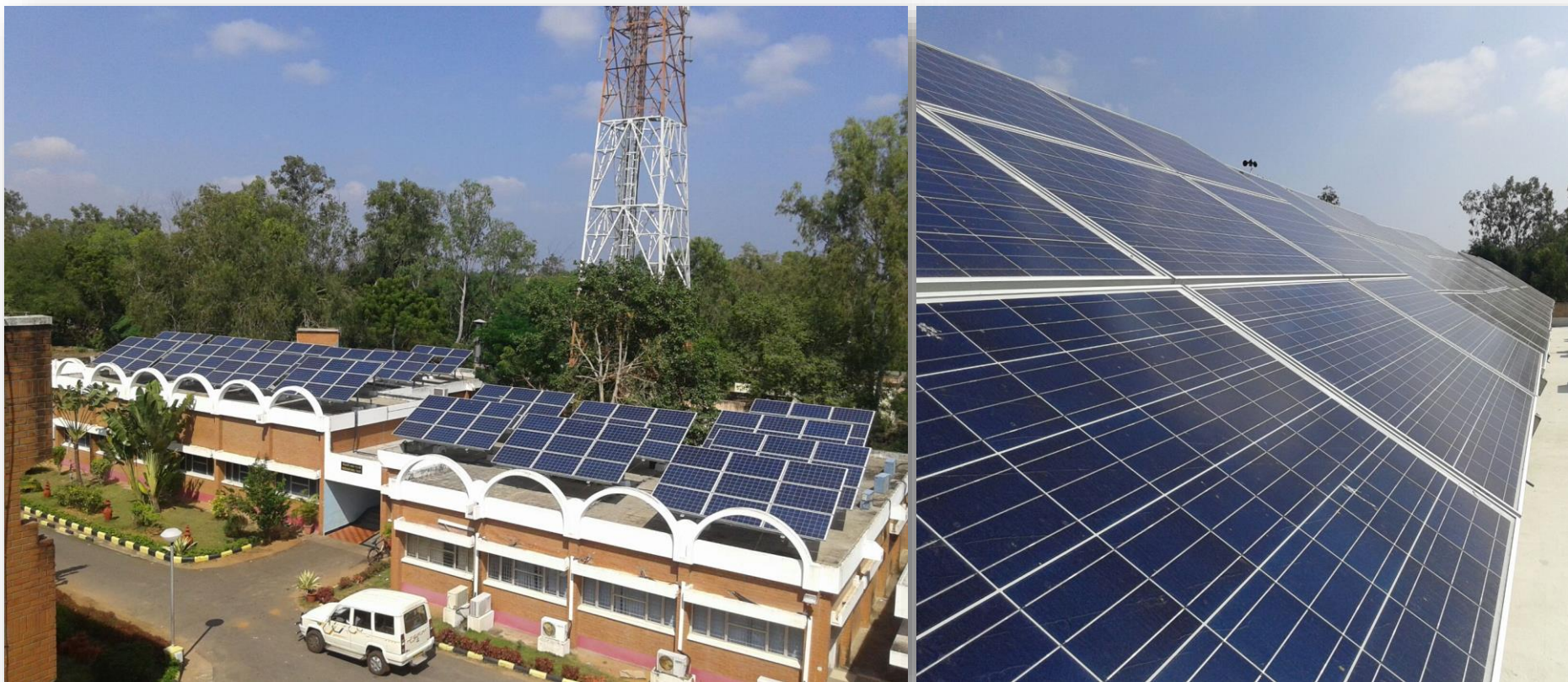
ISRO - 3060 KW SOLAR ROOFTOP INSTALLATION
